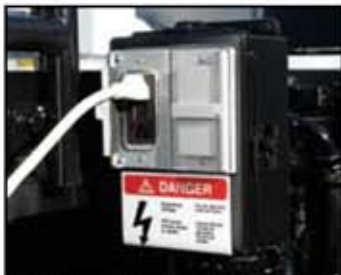
110 Volt outlets for lights or tools.
